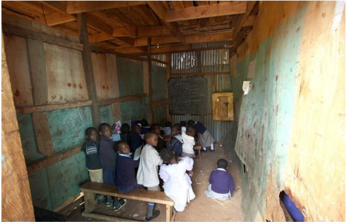
Figure 11 Dilapidated classroom interior
